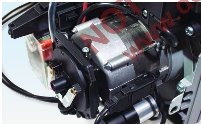
Pressure switch DL mounted on heating boiler
