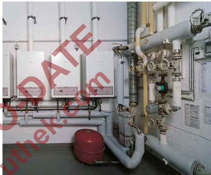
Heating boilers connected in cascade
